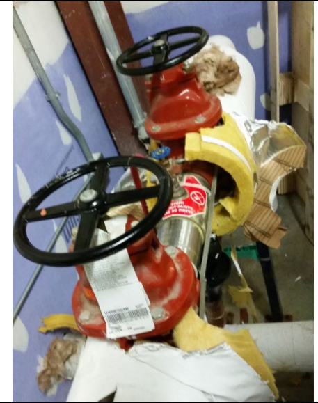
MAIN WATER SHUTOFF (MECH RM)
