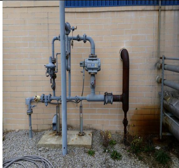
MAIN GAS SHUTOFF (MECH RM EXTERIOR)
