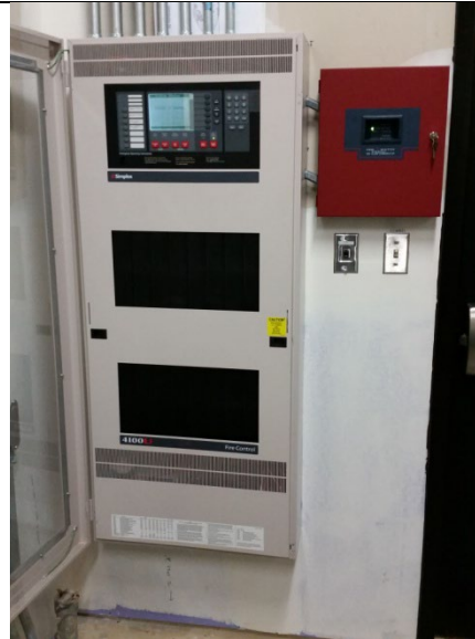
FIRE ALARM PANEL (MECH RM - SIMPLEX)
