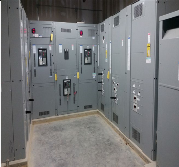
MAIN ELECTRICAL SHUTOFF (MECH RM)
