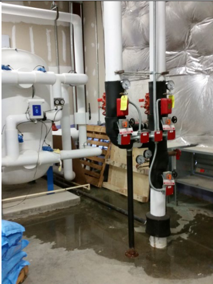
MAIN SPRINKLER SHUTOFF (MECH RM)
